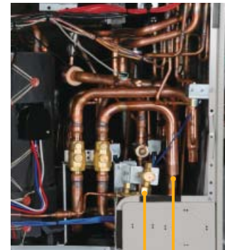
Liquid pipe Gas pipe
